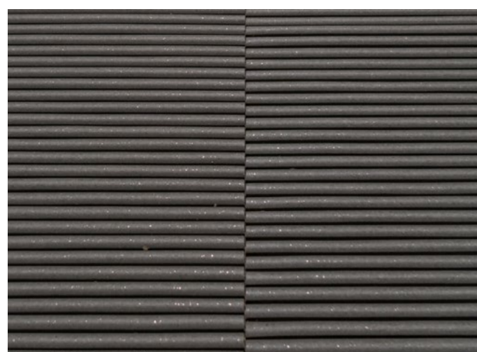
Before: Imperfect rib alignment.
